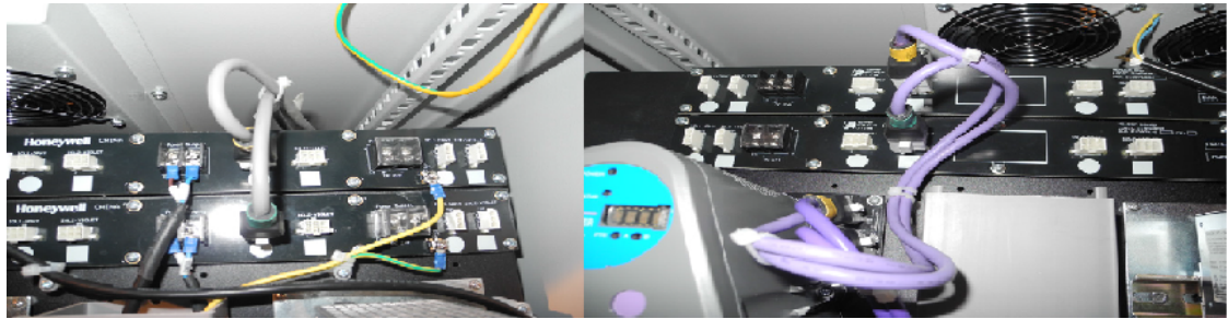
Figure 3: Cabling for the power distribution subsystem
