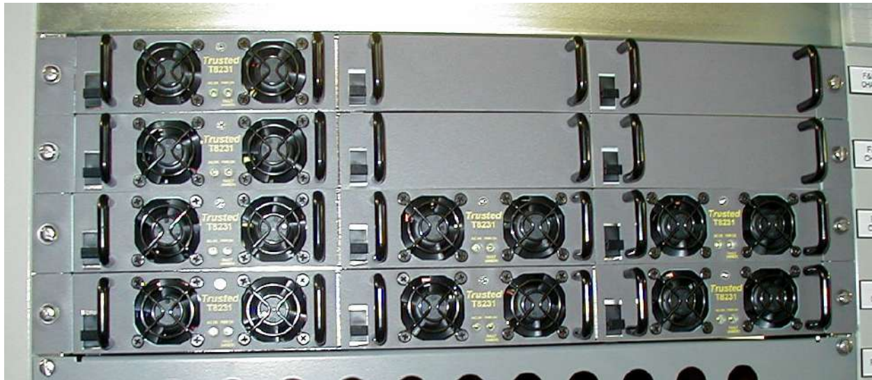
Figure 7-5: Power System (Front View)
